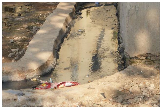
They also observed open gutters, and found that the allowed water to stagnate, creating health risks to local residents.
